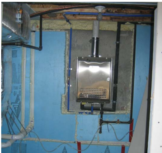
Figure 9. The tankless water heater on the basement wall
