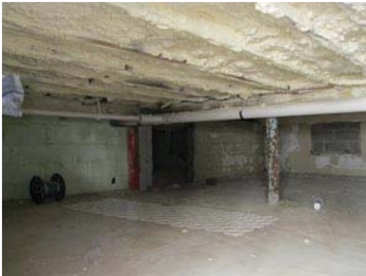
Figure 20. Closed cell spray foam under the first floor. The basement has been filled and topped with a concrete slab to comply with city flood zone requirements.
