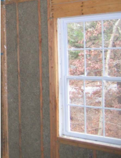
Figure 3. Rock wool insulation
