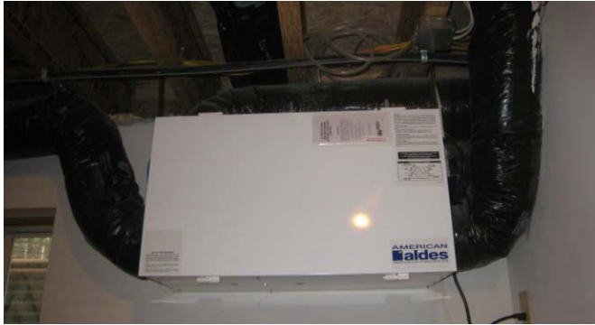
Figure 13. An American Aldes HRV is installed in the insulated basement
