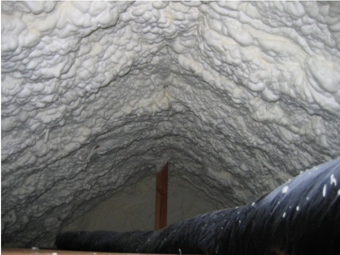
Figure 24. Low density spray foam used to enclose a small area of the attic containing mechanical equipment
