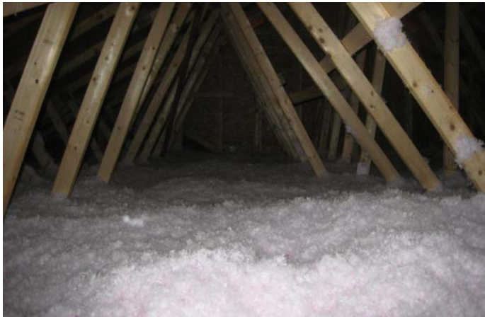
Figure 12. Blown-in attic insulation
