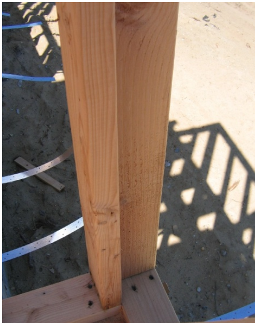
Figure 7. Some advanced framing techniques were used such as at this 2-stud corner
