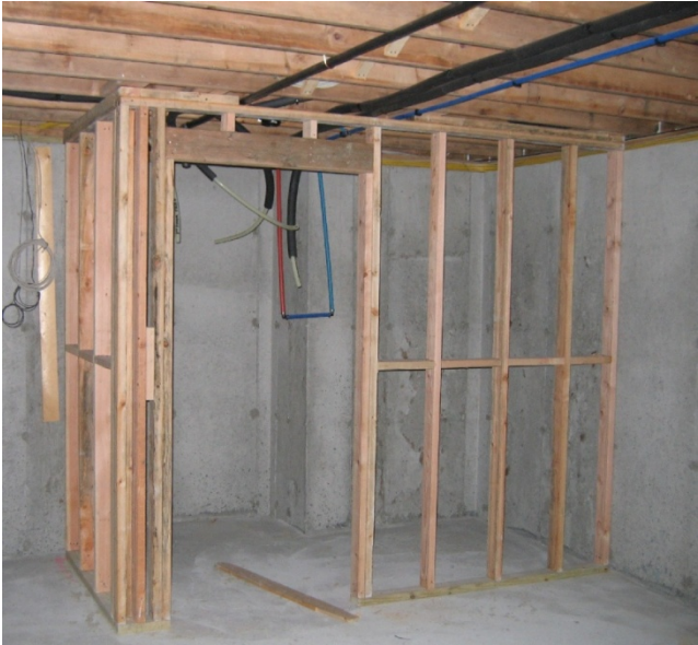
Figure 4. Basement mechanical room framing – the framed and concrete walls were later insulated
