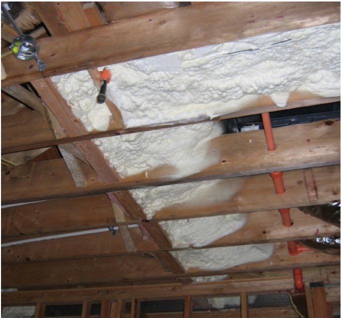
Figure 25. Blocking and spray foam was used to extend the thermal and air barrier through the ceiling joists under the walls enclosing the attic mechanical space
