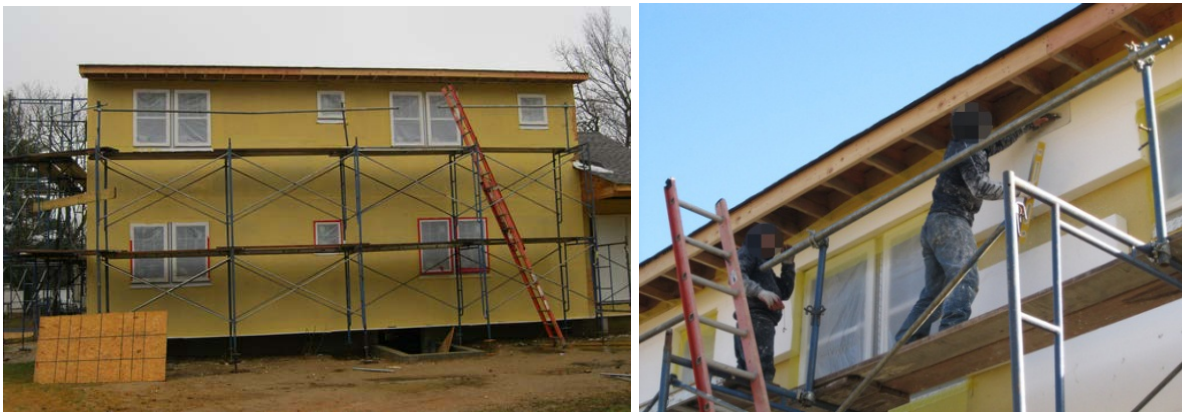
Figure 7. Sections of EPS insulation, 4 in. thick and measuring 2 ft × 4 ft are adhered to the walls. Where necessary the backside of the panels are rasped to conform to irregularities in the substrate wall. The EPS joints are smoothed out.
