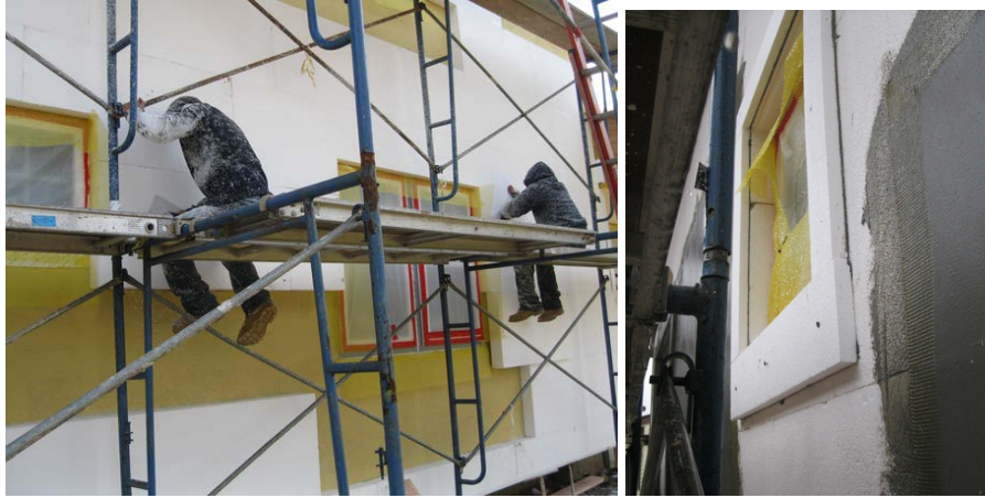
Figure 8. EPS panels are placed around the new windows; an additional 1-in. thick by 4-in. wide layer of EPS is used to form window trim. Other applied shapes can be used to create architectural forms as desired.
