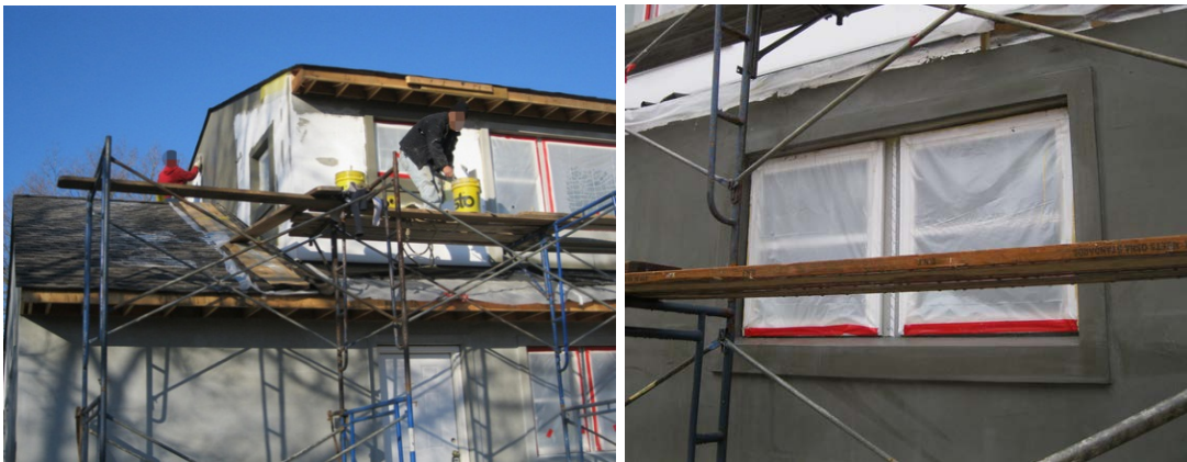
Figure 10. The basecoat is applied over the formed window trim and edges of the EPS panels, embedding the yellow mesh around windows and other penetrations.
