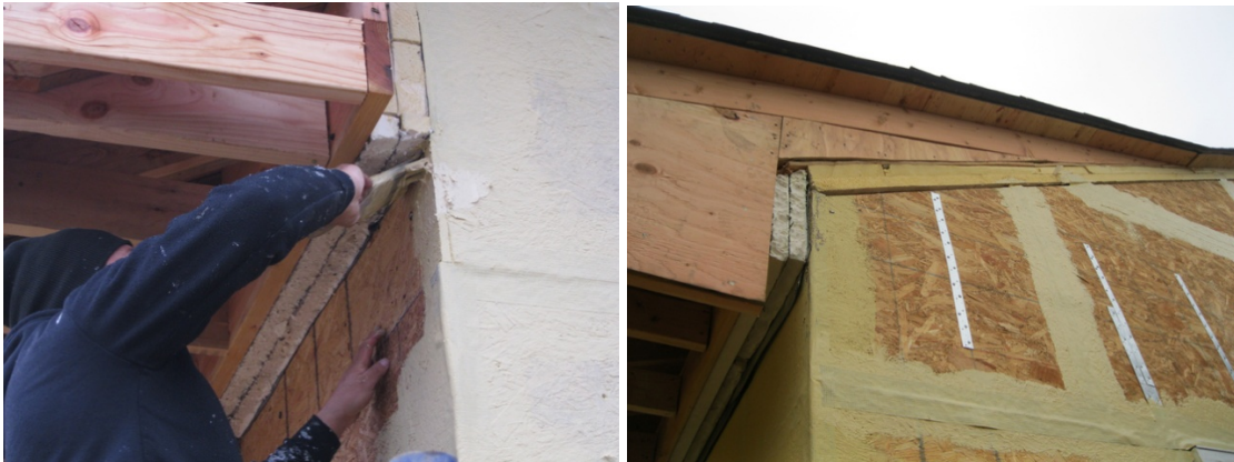
Figure 5. A liquid water resistive coating is brushed onto the sheathing; a layer of reinforcing mesh is embedded into the coating at the sheathing joints.
