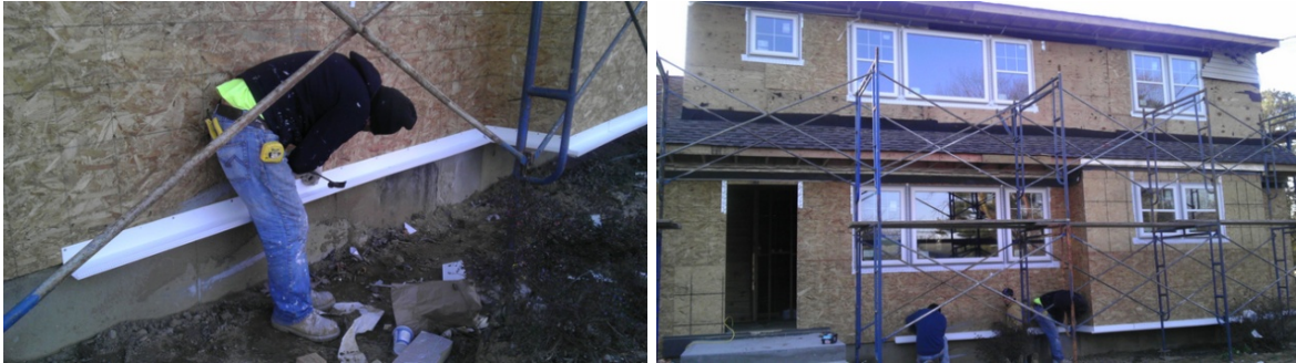
Figure 4. After scaffolding is set up a bottom track is attached to the base of the sheathing to accept the bottom of the EIFS.
