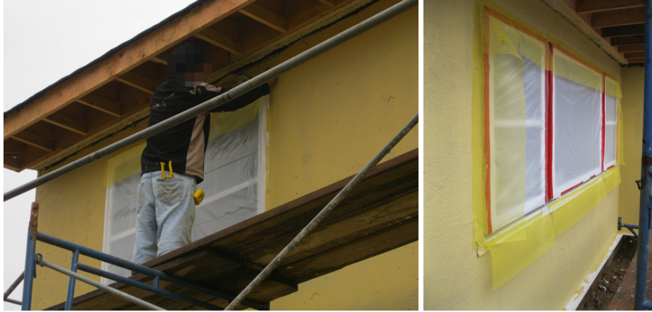
Figure 6. After the coating is complete, more reinforcing mesh affixed around the newly installed windows; it will be used to wrap the edges of the insulation.
